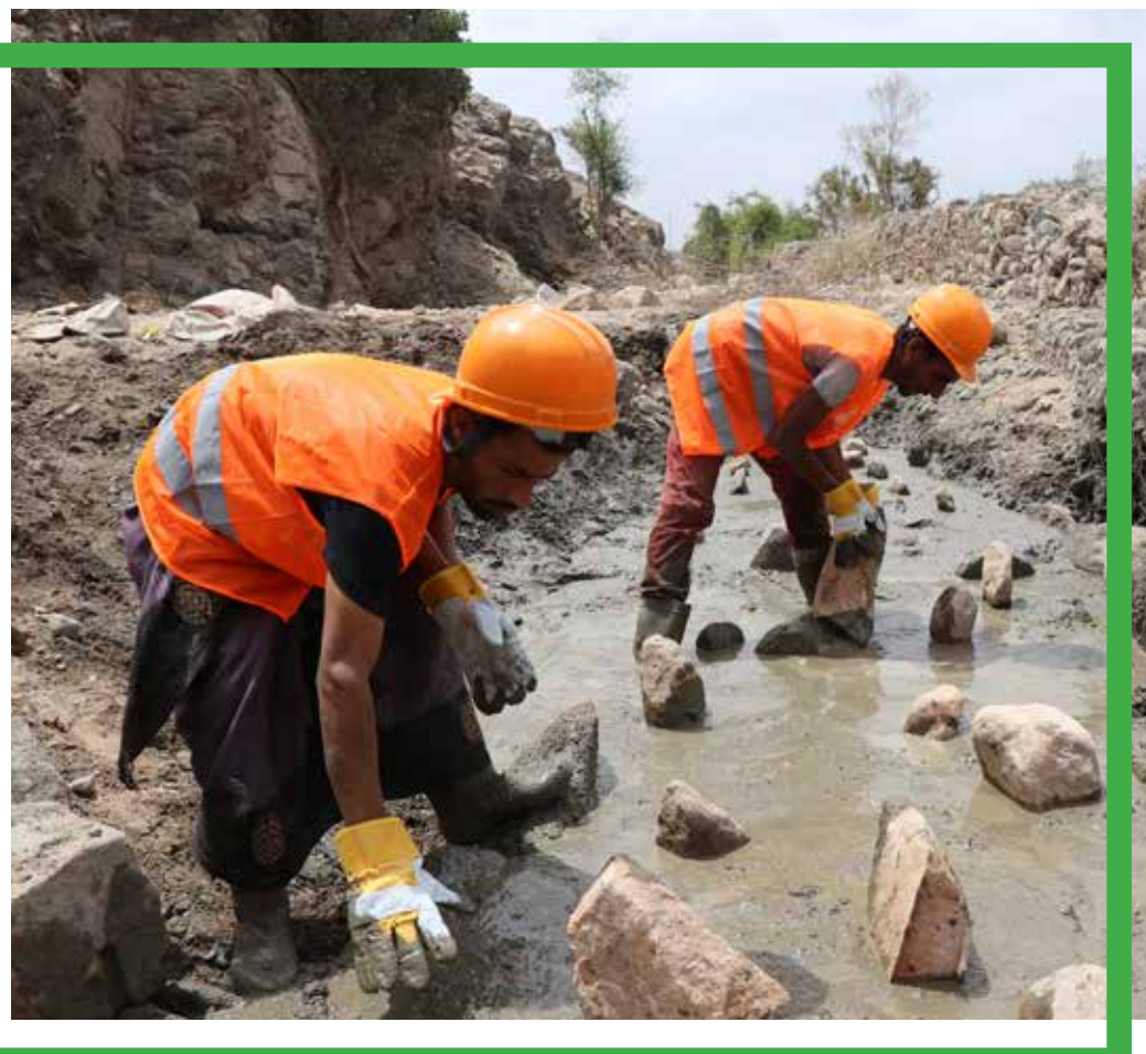
Implementing gabions to divert torrents in the village of Al-Thameer - Radfan - Lahj
